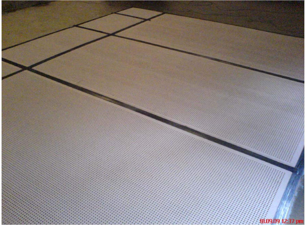
Figure 3 – Sample 2, 5mm round perforated fibre cement sheeting installed on test room floor
